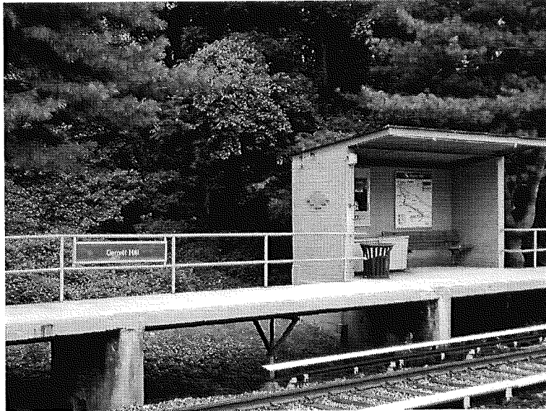
Unattractive concrete block shelters with inadequate waiting area
