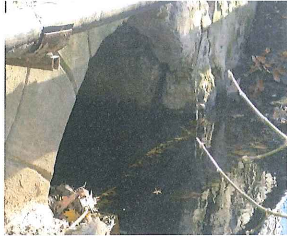
Failing Upstream Headwall in South Barrel
