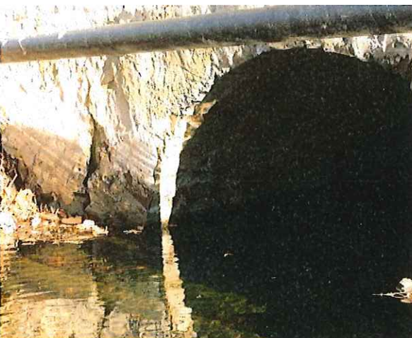
Spall and Missing Stones in Upstream Masonry Headwall of North Barrel
