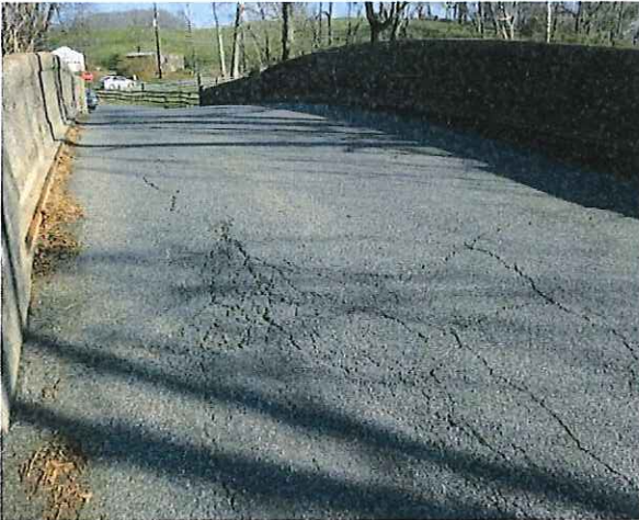
View of Pavement – Cracks throughout
