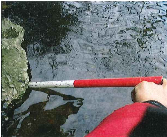
2' Undermining under Wing B Apron
