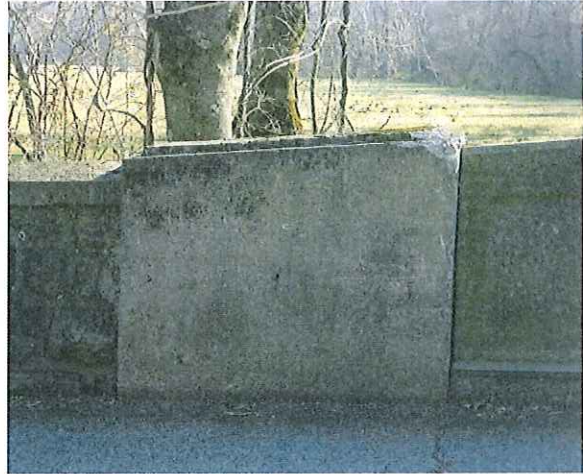
Spalls in Bridge Barrier
