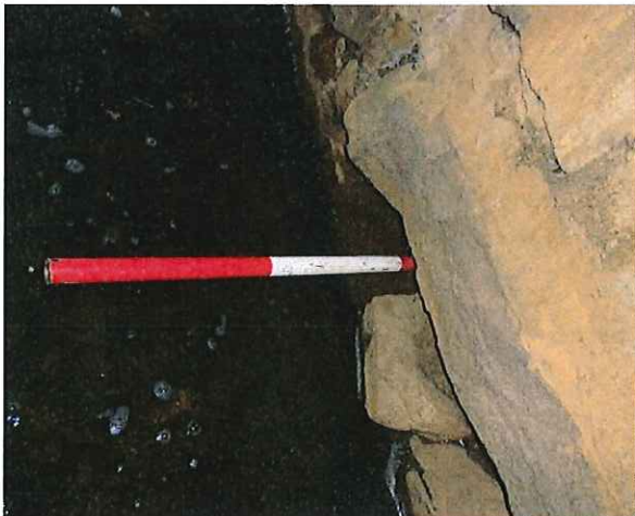
2' Deep Void in North Abutment
