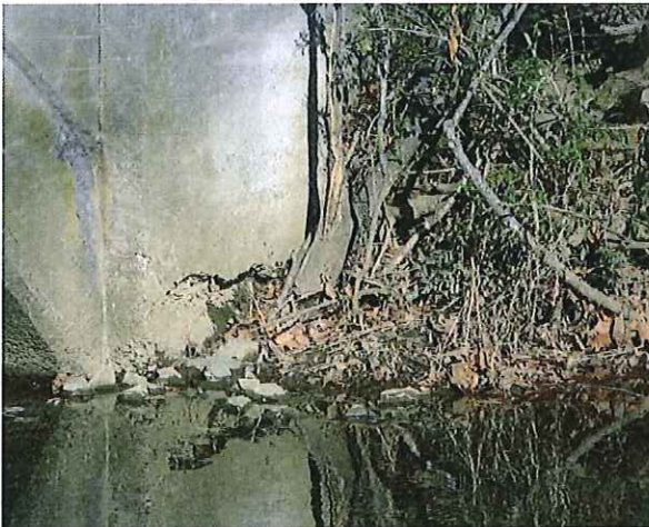
Large Spall at Bottom of Southeast Wingwall
