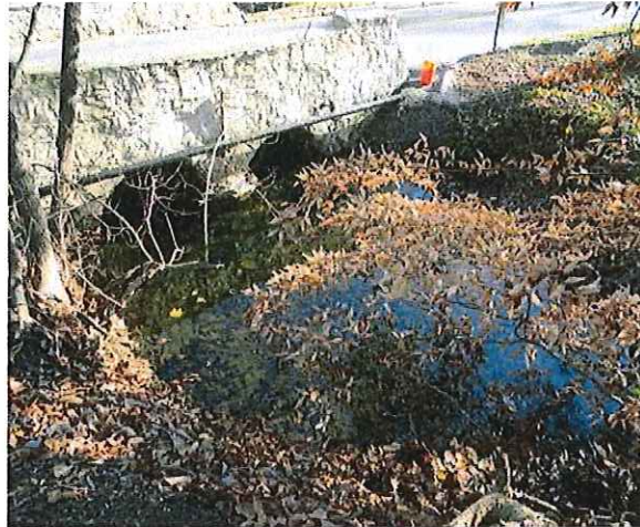
Large Scour Hole/Pond formed at Culvert Inlet
