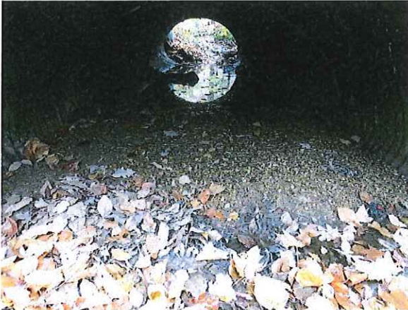
West Pipe with Heavy Silt Built-up
