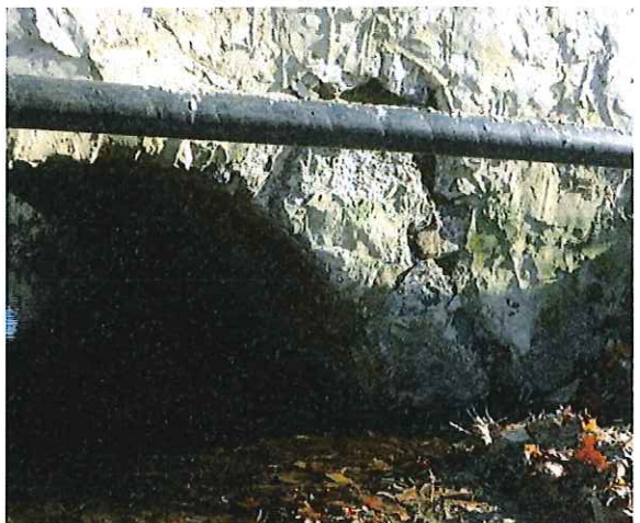
Spall and Missing Stones in Upstream Masonry Headwall of South Barrel
