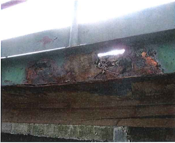
100% Loss in Web of North Stringer
