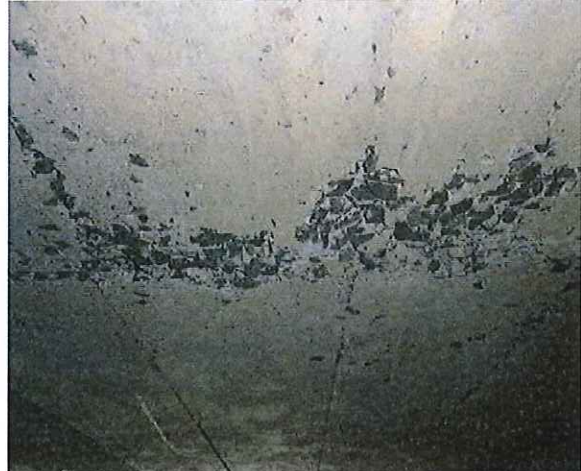
Honeycombing and Exposed Aggregate
