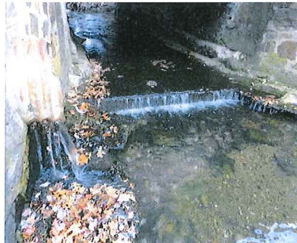
Large Scour Hole at end of Culvert
