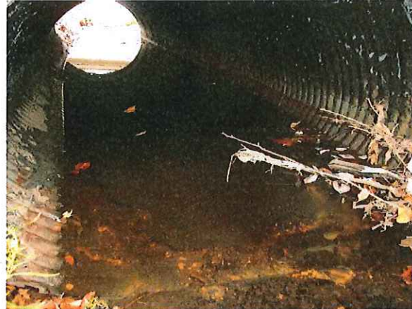
East Pipe with Apparent Heavy Rust
