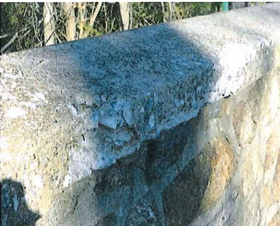
Spalls in Concrete Cap of Wingwall Barrier
