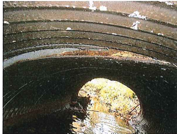
Upstream portion of East Pipe shows Excessive Deformation & Separation from Abutting Section
