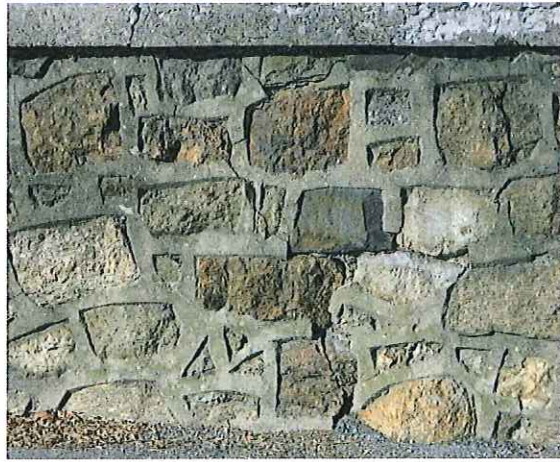
Cracks in Wingwall Barrier
