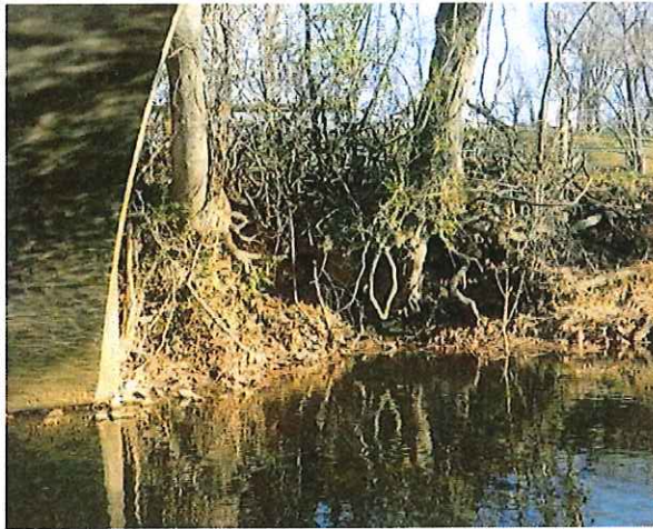
Bank Erosion with Exposed Tree Roots in Bank of Southeast Corner of the Bridge
