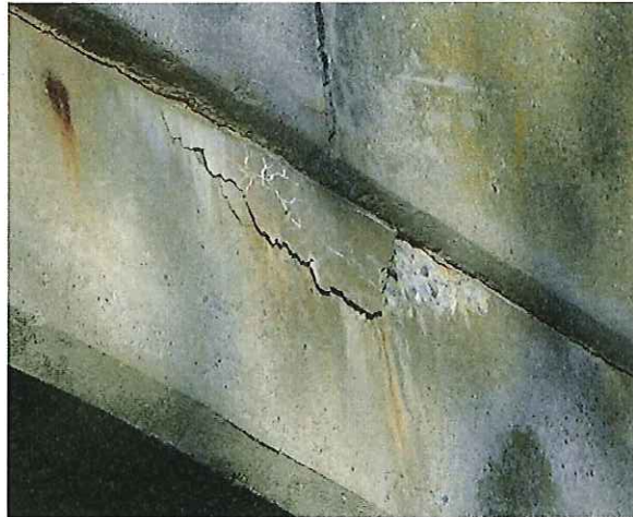
Surface Spall in South Fascia of Arch Barrel
