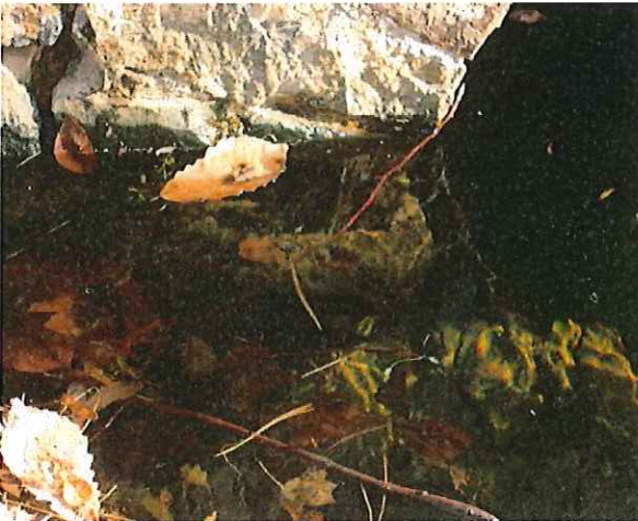
Scour and Exposed Footing at Upstream North Barrel
