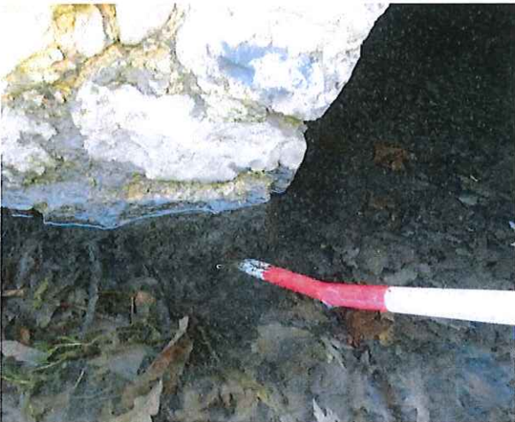
1'-0" Undermining at Outlet
