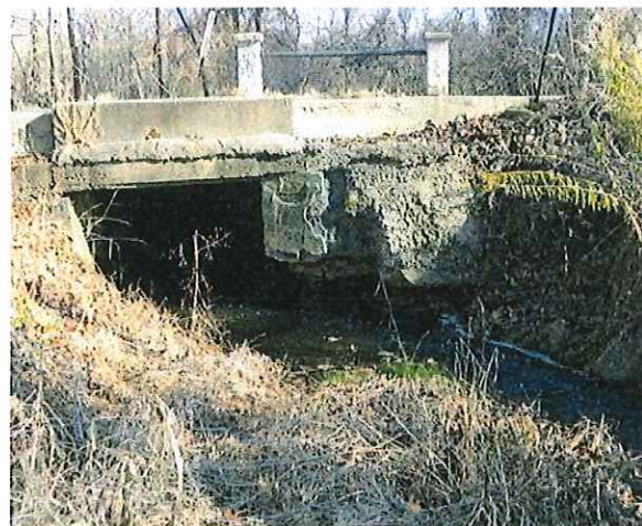
Upstream Elevation. Note Stream Flow Entering the Culvert with a Sharp Skew and Skew of the Culvert
