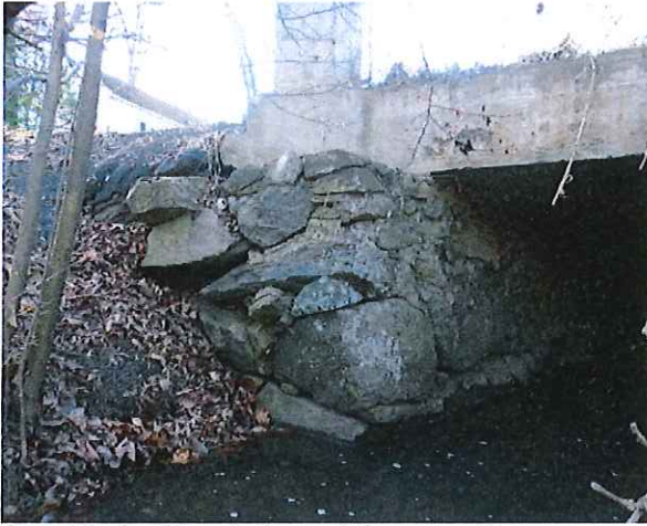
East End of South Stone Masonry Abutment, Note Large Stones with Missing Mortar Joints
