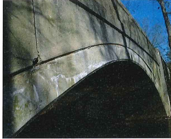
Small Spall in South Spandrel Wall and Fine Map Cracks with Efflorescence in South Fascia of Arch Barrel
