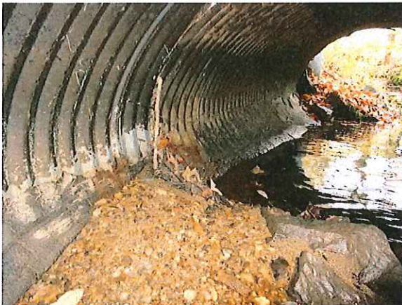
Misaligned/Distorted West Pipe Shows Loss of Fill Material
