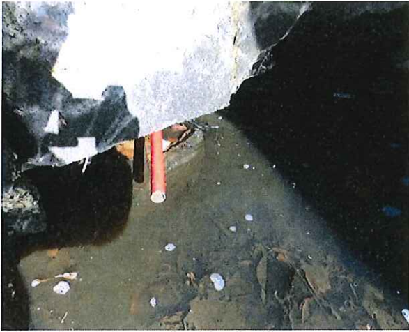
4' Undermining under North Abutment of Inlet Structure
