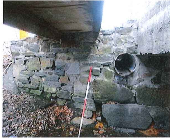
Missing Stones and Mortar Joints in Wing A
