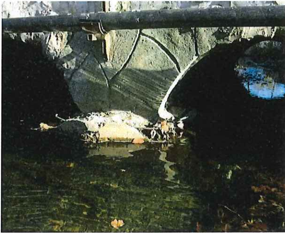
Undermining and Spall in Upstream Pier Footing
