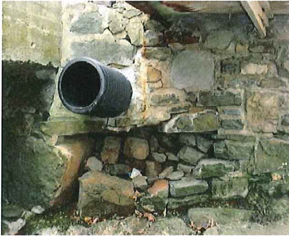
Missing Stones and Undermining in Wing D
