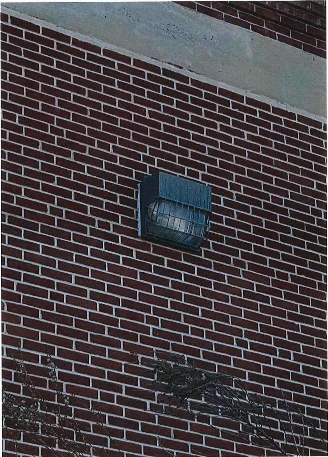
Site photo, typical PECO/SEPTA substation wall mounted luminaire
