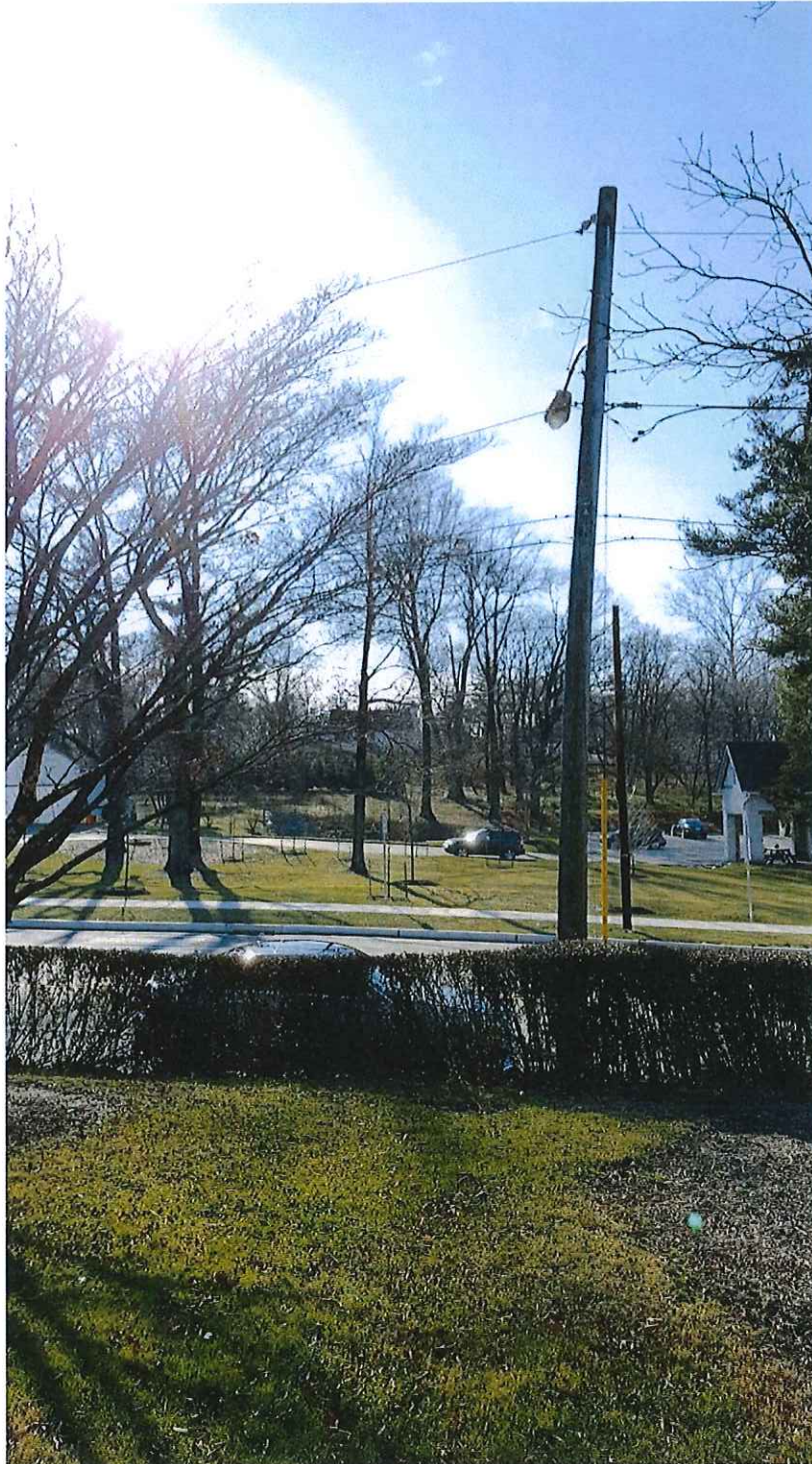
Site photo, pole mounted street light at Lancaster Avenue
