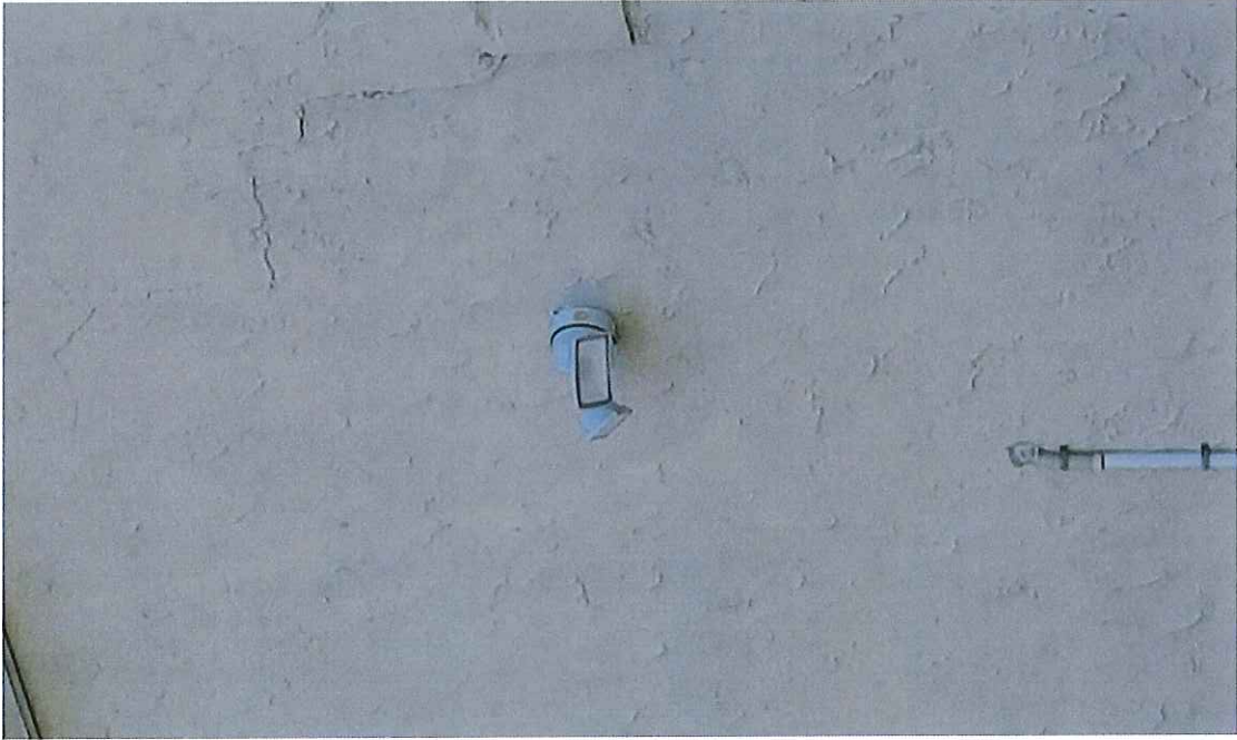
Site photo, restaurant luminaires
