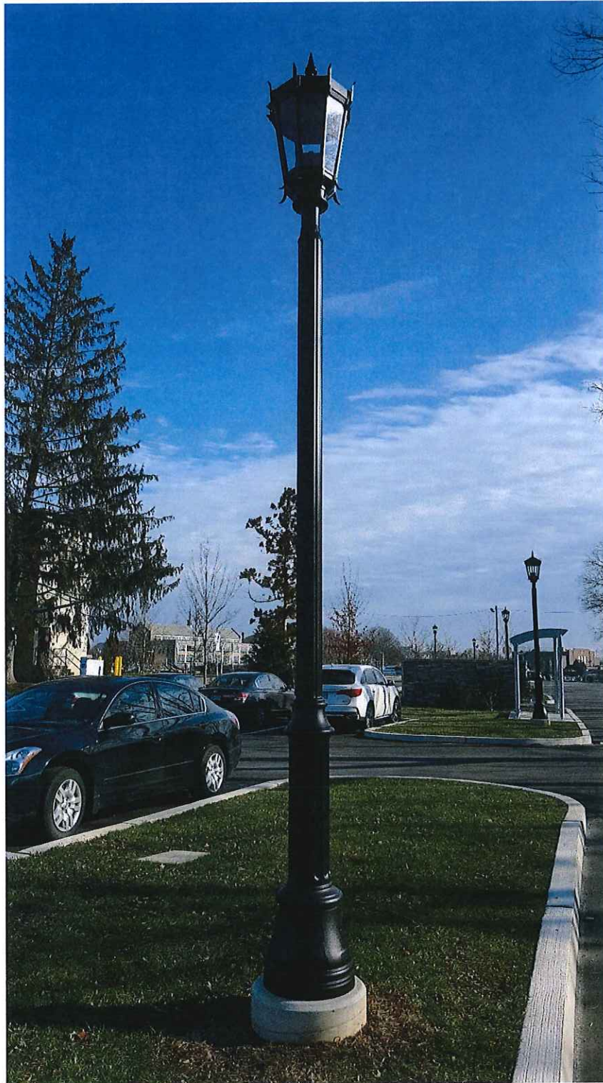
Site photo, typical WLAPF luminaire with 2" shielding band
