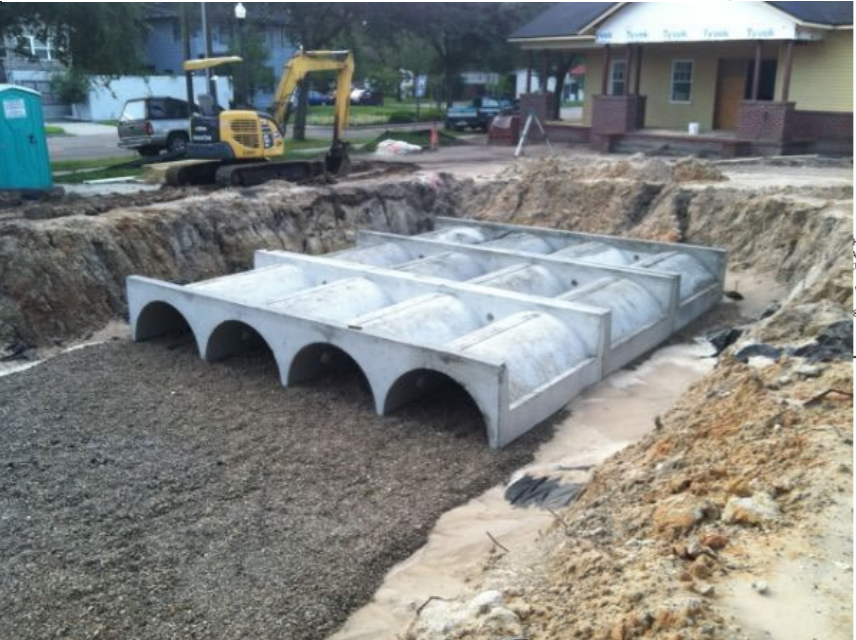
Subsurface Stormwater Storage
