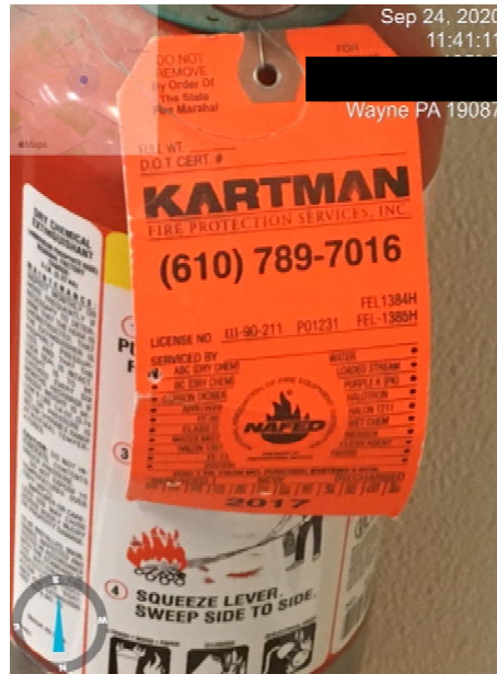
Out of Date Extinguisher
